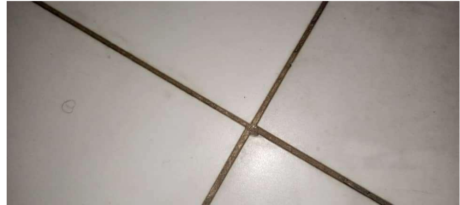
Pic showing: Toilet tiles that need proper grouting.
