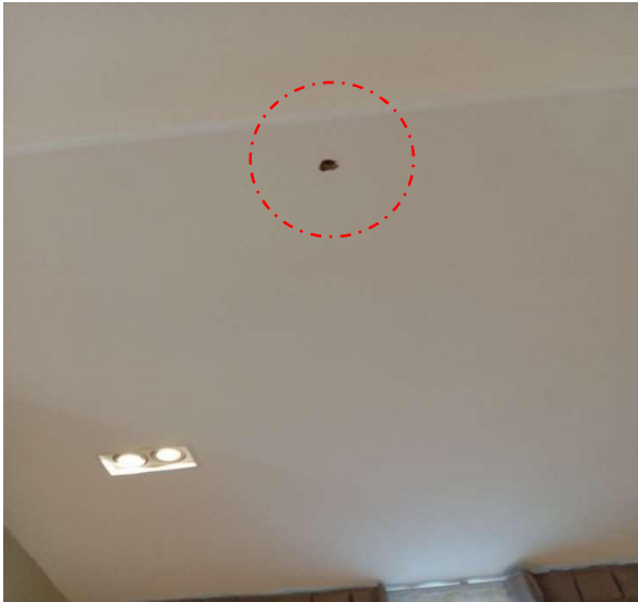
Pic showing: The presence of punctured holes in the plaster of Paris (POP) ceiling board may suggest deficiencies in the quality of finishing, workmanship, and board thickness.
