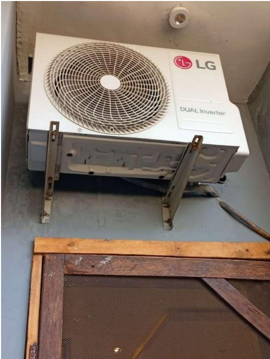
Pics showing the outdoor unit of the air conditioning system discharges water at the rear exit door, which may be an inadvertent occurrence.
