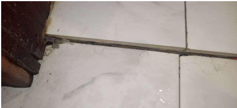
Pic showing several tile joints with poor sealing and workmanship.
