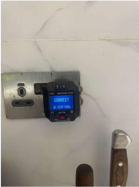
Picture showing correct voltages in the socket
