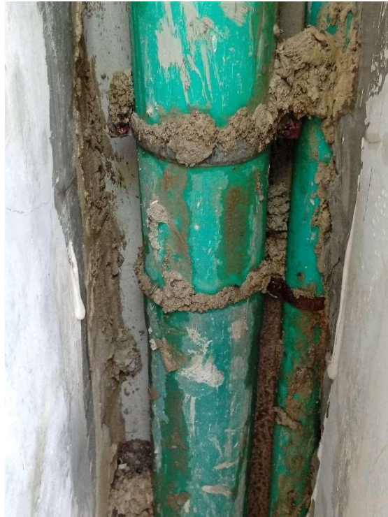
Pics showing an extremely damped 4'' pipe and duct wall, mainly observed to be leaking from the union connector on the upper floor.
