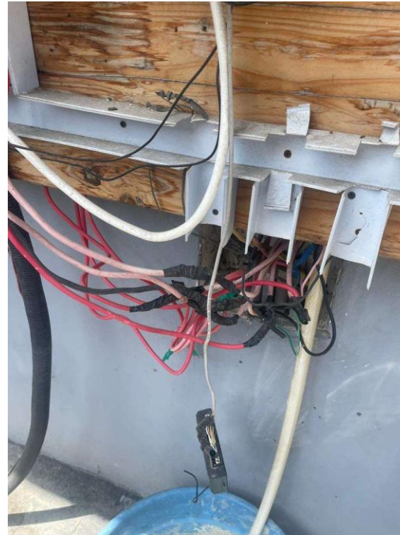
Picture showing rough termination of cables externally
