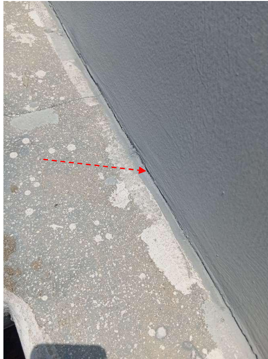
Pic showing visible cracks along the edge of the roof slab and wall, which can be attributed to a failure to achieve proper bonding and a deficiency in waterproofing measures to prevent water ingress.
