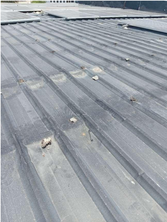
Pics showing a dent on the roofing sheet because of footsteps on the roofing sheet, mainly during solar panel installation.
