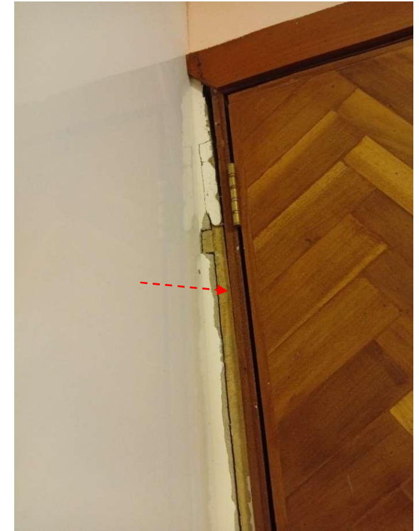
Pic showing: There exists an uneven clearance between the door and the frame, indicating that the door may be misaligned, either being out of plumb or exhibiting warping.
