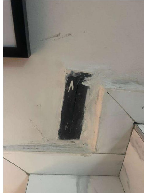
Picture showing damaged step light
