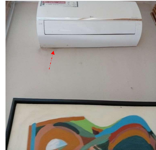
Pic showing: Mechanical Fault on the AC Unit, water leakage under the AC unit.
