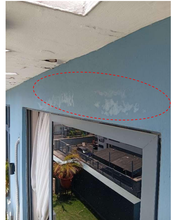
Pic showing: Visible dampness efflorescence beneath the master bedroom concrete slab wall.
