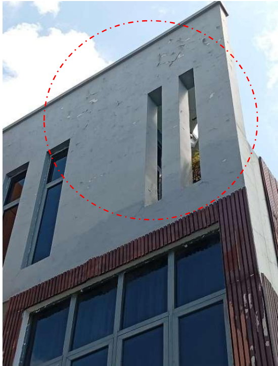
Pic showing: Widespread peeling of the exterior paint layer, especially on the upper facade. Indicates loss of adhesion between paint and substrate.
