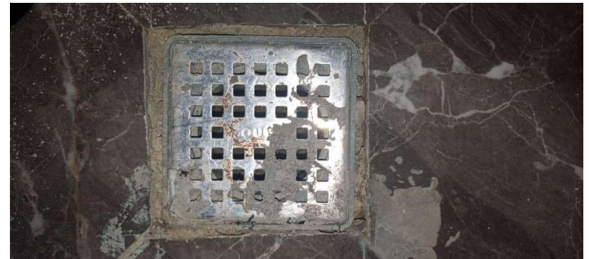
Pic Showing: Corroded floor drain with deteriorated sealant around the drain frame, indicating maintenance and resealing required.
