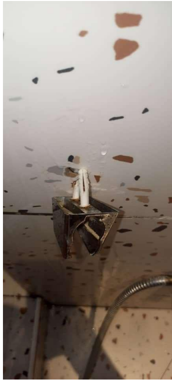
Pic showing: Hand shower hanger displaced, this should be properly fixed back to the wall to prevent future home hazards.
