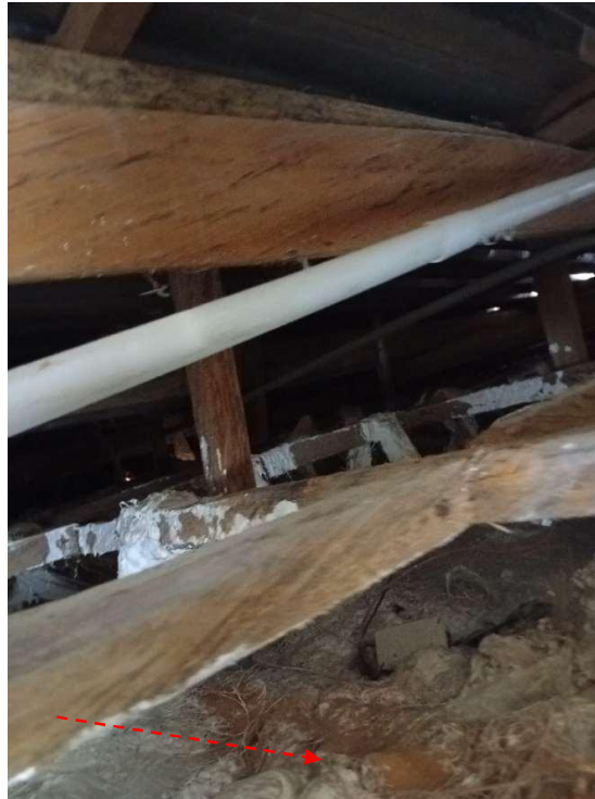
Pic showing: The wood members of the roofing systems being attacked by termites, causing the wood to deteriorate and lose its strength.
