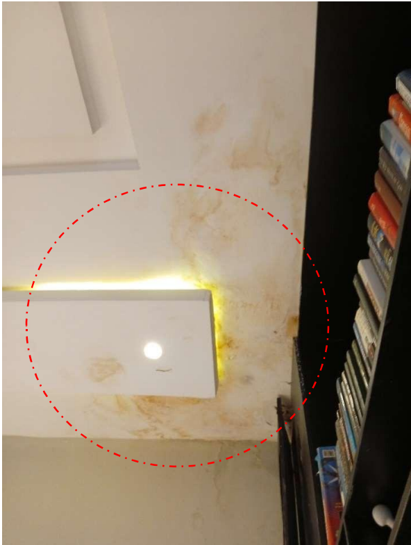
Pic showing: Pop discoloration due to water leakage from the master bedroom open terrace floor.
