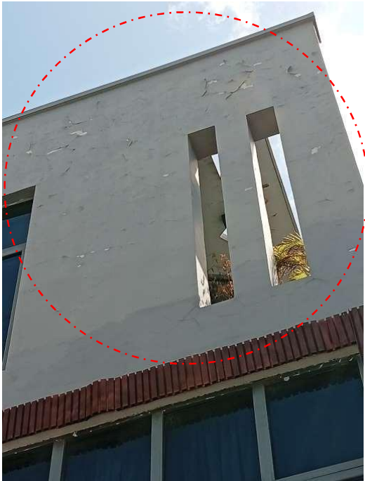
Pic showing widespread peeling of the exterior paint layer, especially on the upper facade.
