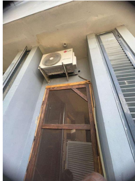
Picture showing a faulty light fitting and AC dripping water directly to the floor
