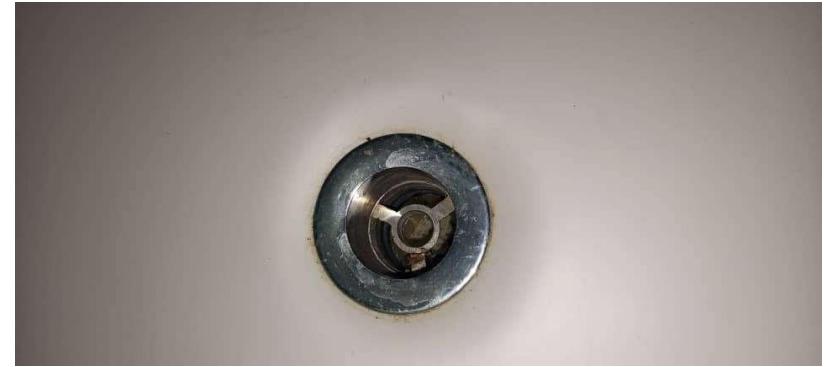
Pic Showing: Jacuzzi bath pressing no waste that needs to be replaced.
