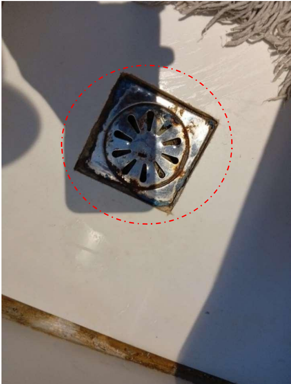
Pic showing: The floor drain is positioned lower than the surrounding tiles, which allows water to seep into the floor. This can lead to dampness in the walls as moisture accumulates over time.
