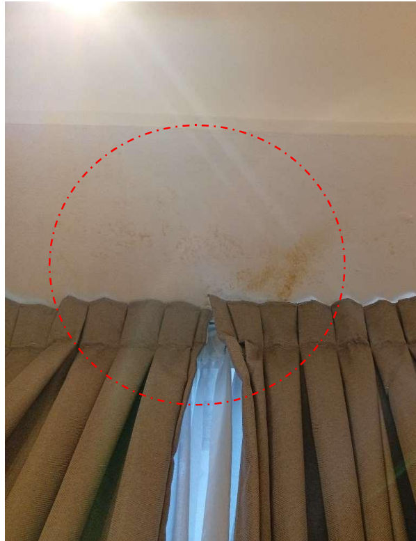
Pics showing: Pop discoloration due to water leakage from the master bedroom open terrace floor.
