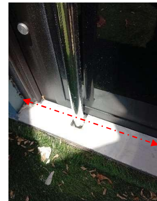
Pic showing: Improper door sealing and roof cover to prevent rainwater seepage during heavy downpour.
