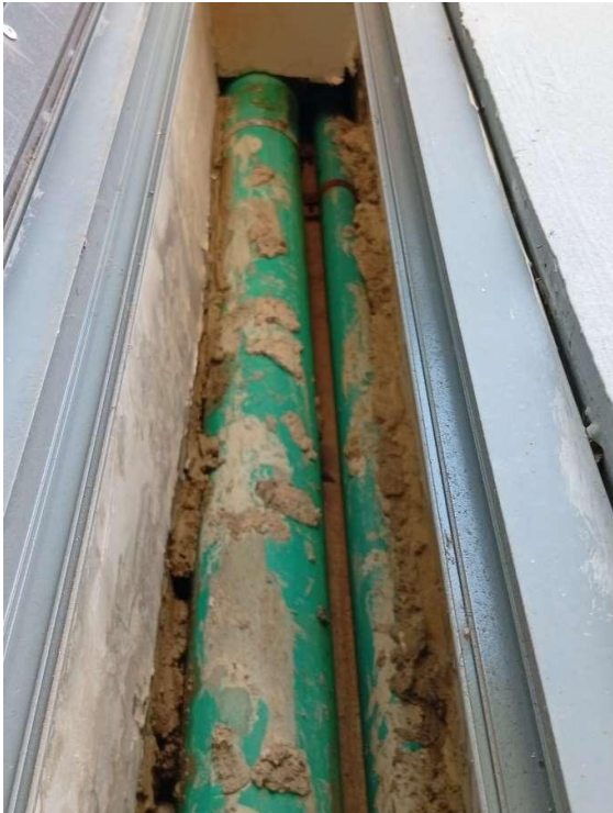
Pics showing an extremely damped 4'' pipe and duct wall, mainly observed to be leaking from the union connector on the upper floor.
