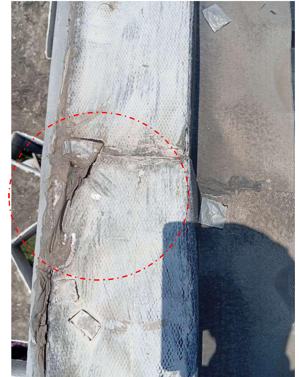
Pic showing repaired roof cap flashing; however, it still contains porous openings that may permit water infiltration into the adjacent block wall.
