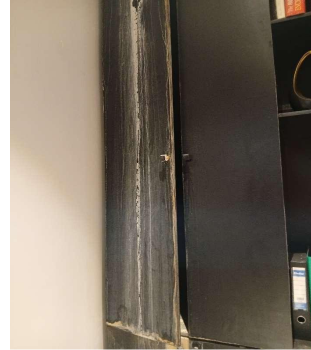
Pic showing: Damaged office wardrobe due to water leakage from the master bedroom open terrace floor.
