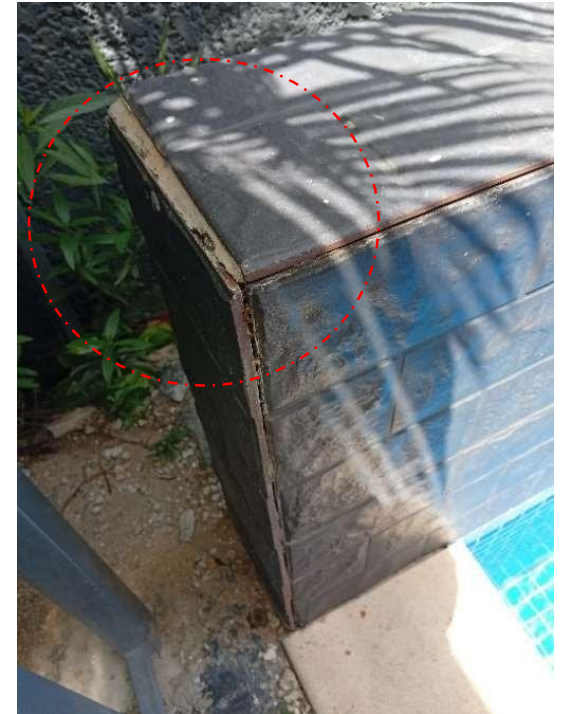
Pic showing: Swimming pool tiling reflecting shoddy workmanship.
