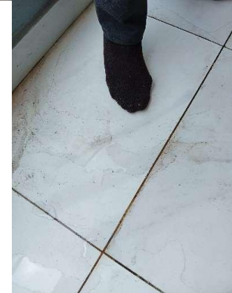
Pic showing water spillage from the outdoor AC unit, thereby creating constant water stagnation on the terrace floor.
