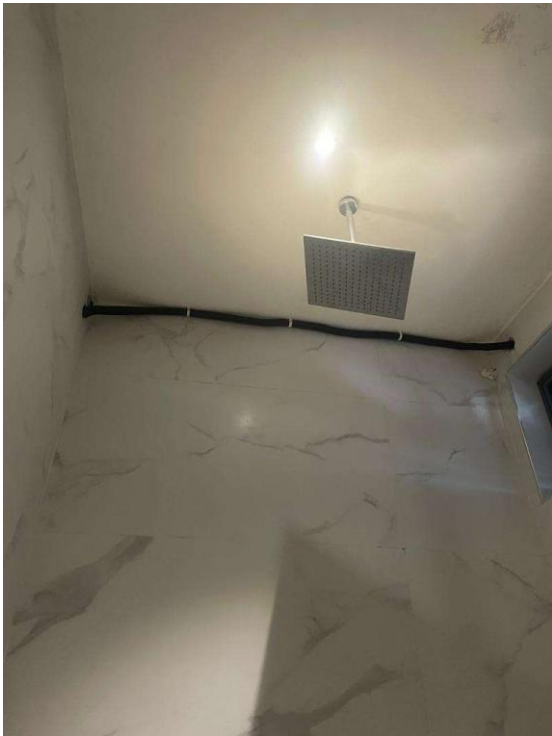
Picture showing illumination blocked by the shower head
