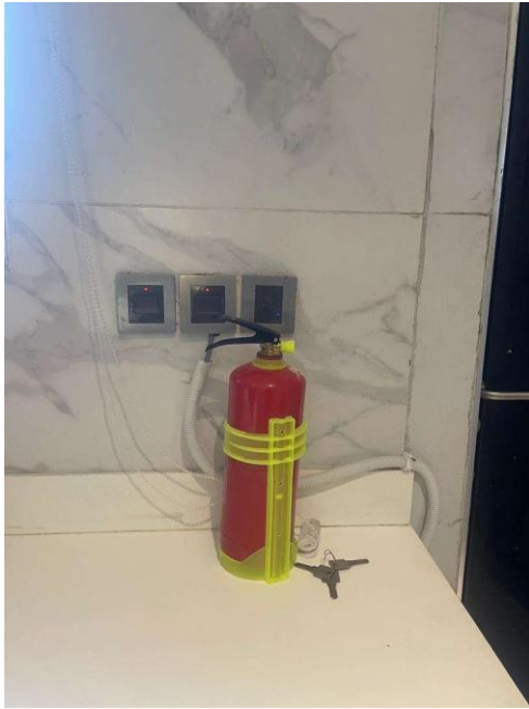
Picture showing properly aligned switches and a fire extinguisher
