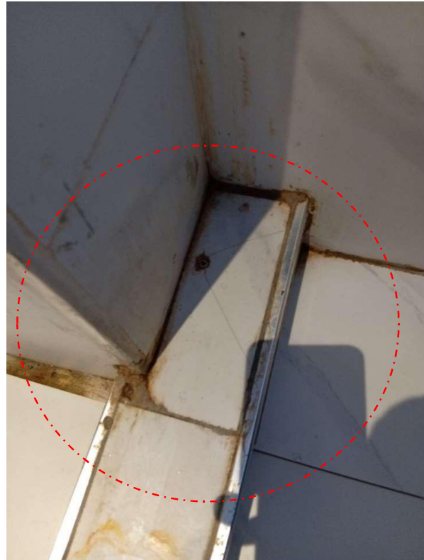
Pic showing: Improper grouting of tiles, mainly along the floor and wall edges, which can lead to dampness of the wall
