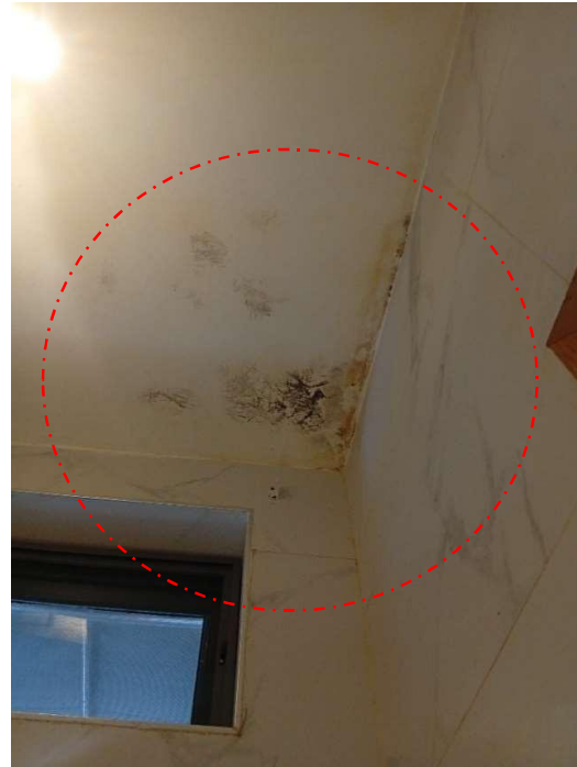
Pic showing: The ceiling exhibits noticeable discoloration, characterized by blackish stains and spots where the pop ceiling material has degraded.
