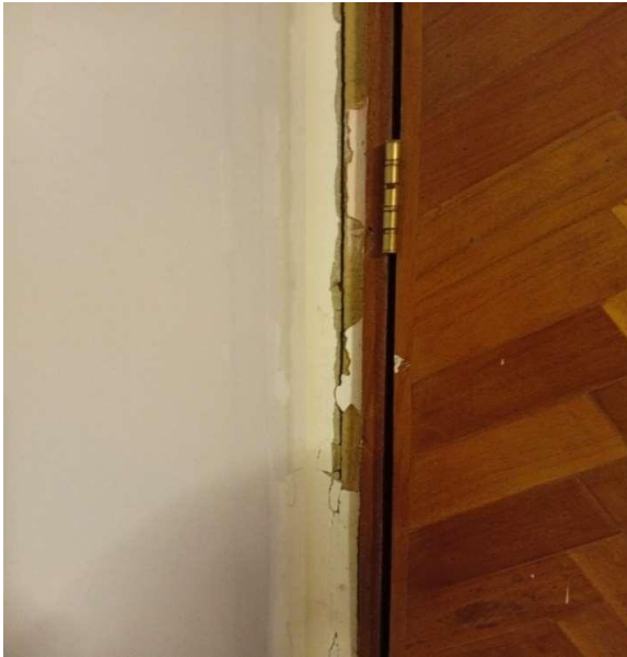
Pic showing: Improper use of wooden doors at toilet entrance, water coming from the bath area can get the door soaked, causing damage to the wooden door.
