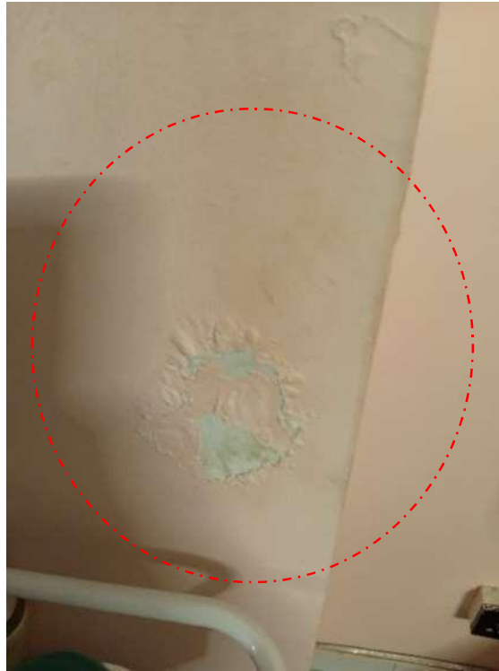
Pic showing an image illustrating a significant concentration of dampness, accompanied by extensive peeling and flaking of finishes, which have been caused by water intrusion from the bathroom.
