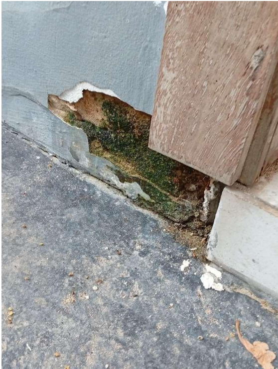
Pics showing flaky walls from base foundation attributed to severe rising damp.
