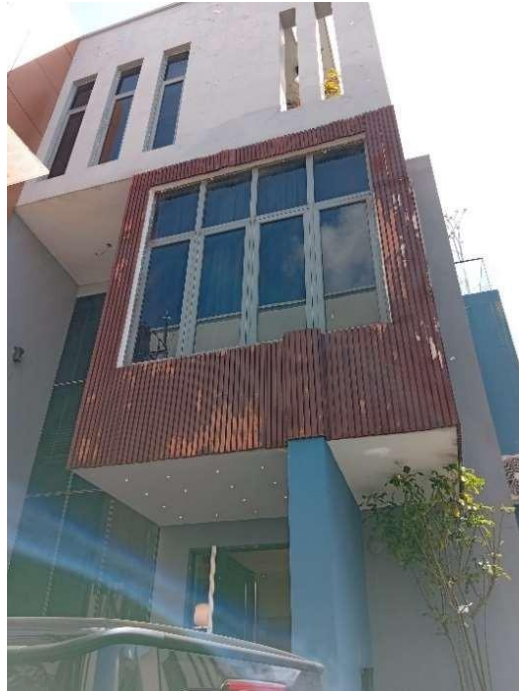
Pic showing the exterior cladding fluted panels are all worn out due to severe weather conditions, causing the building to lose its aesthetic value.
