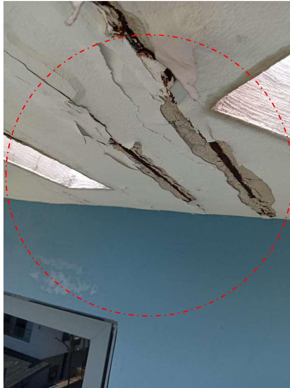
Pic showing: The exposed deterioration of steel reinforcement rebars is attributable to insufficient concrete cover beneath the flooring.
