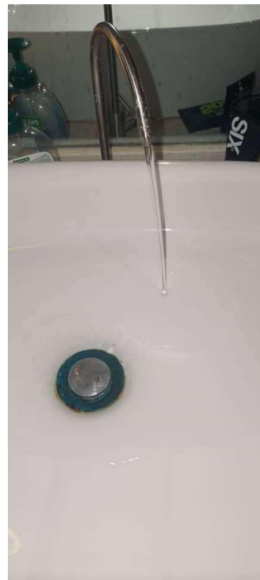
Pic Showing: Hand basin tap with low pressure.
