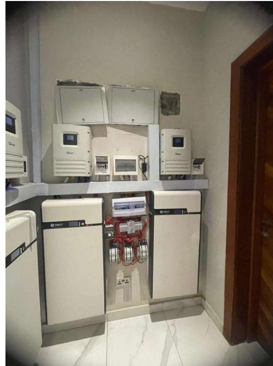
Picture showing an inverter installation without any extinguisher ball.
