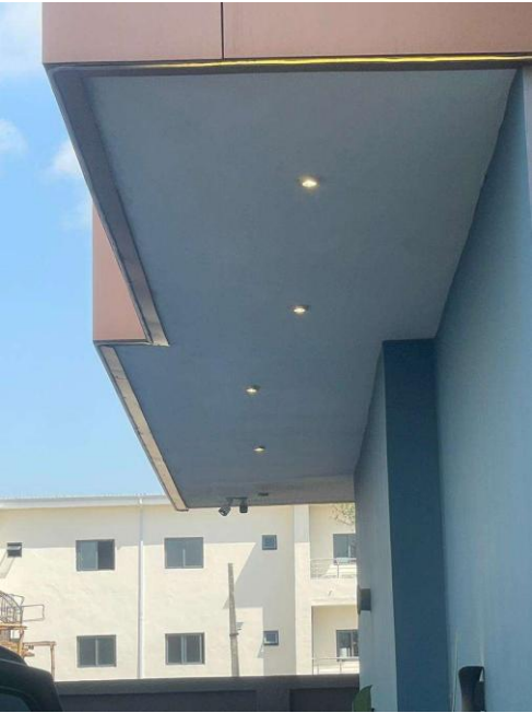
Picture showing a properly installed CCTV camera externally
