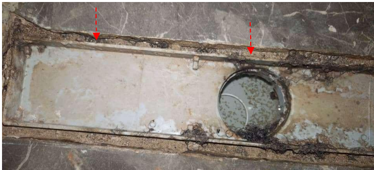
Pics showing the displaced drain outlet needing to be cleaned and sealed properly.
