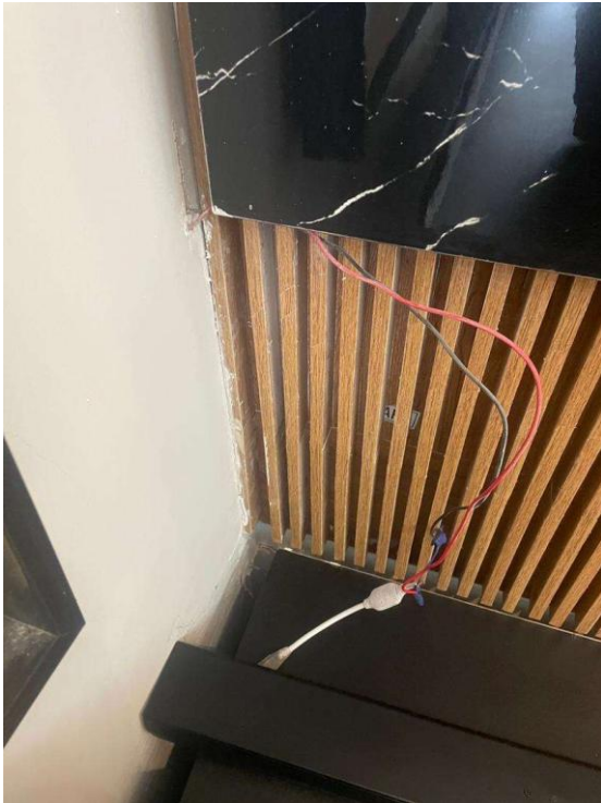
Picture showing an exposed cable for a proposed air-conditioner in the bedroom
