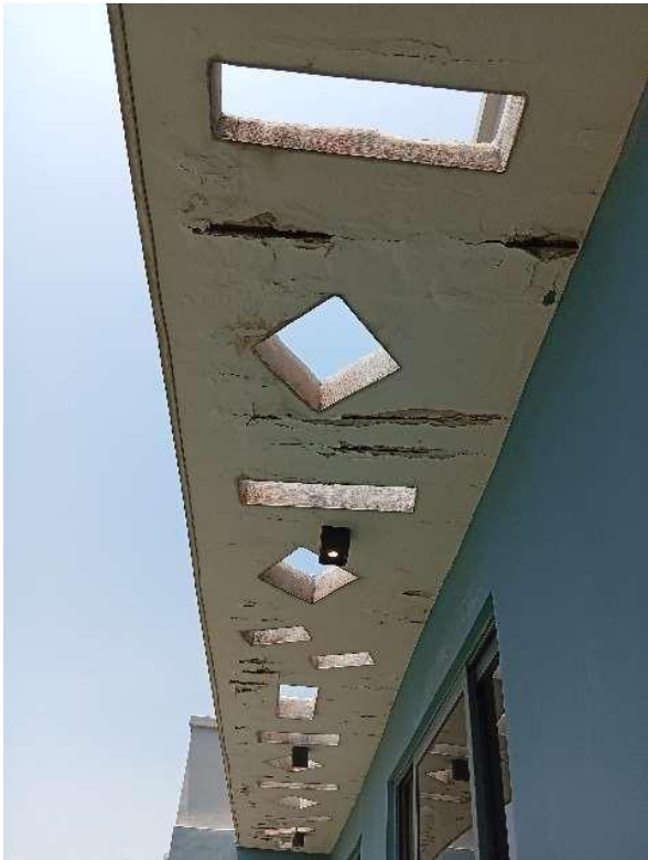
Pic showing: Badly damaged spalling on the concrete slab covering of the open terrace of the master bedroom.
