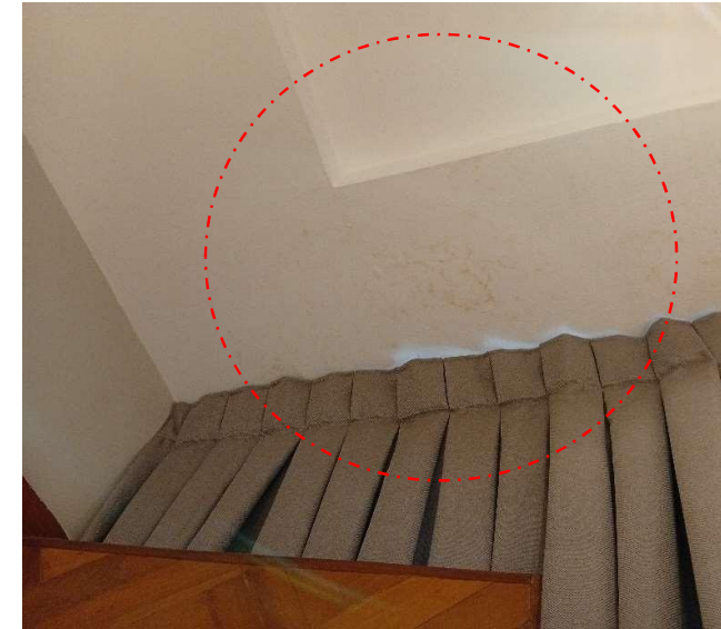
Pics showing: Pop discoloration due to water leakage from the master bedroom open terrace floor.
