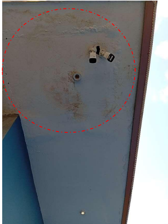
Pic showing: Visible leakage on the cantilevered floor deck, with signs of discoloration from water ingress on the terrace.
