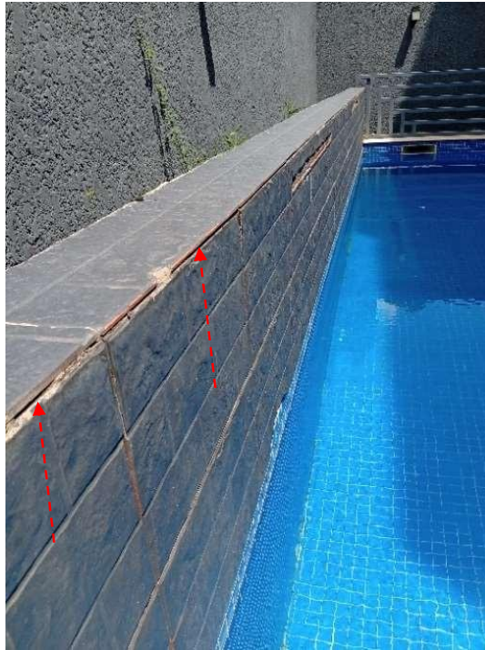
Pic showing: Swimming pool tiling edges not properly sealed, reflecting shoddy workmanship.
