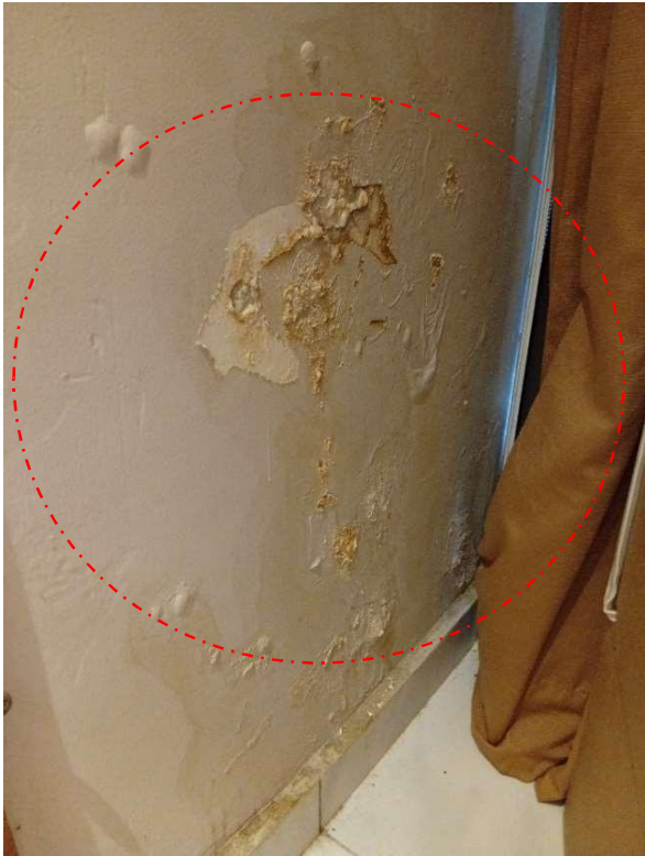
Pics show a severely damp wall with extensive peeling and flaking of paint caused by water ingress from improper tile grout from the toilet behind.
