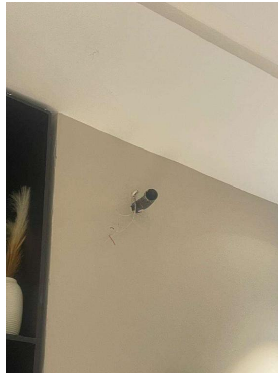
Picture showing an exposed cable intended for an air-conditioner in the office
