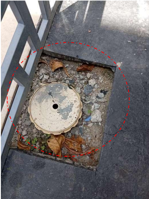
Pic showing uncovered opening on stamped flooring, which may result in water creating a void beneath.
