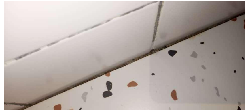
Pic showing: Toilet floor tiles with visible poor grouting on floor and wall tiles.
