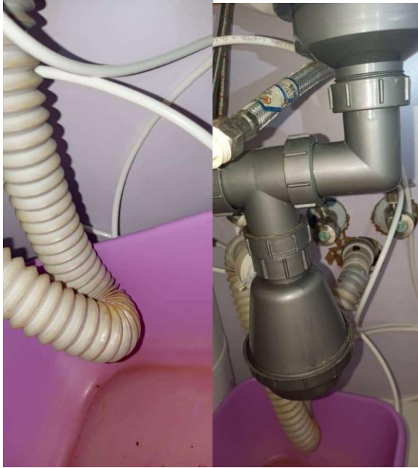
Pic showing: under-sink plumbing showing drainage connection and evidence of suspected leakage requiring plumbing repair.
