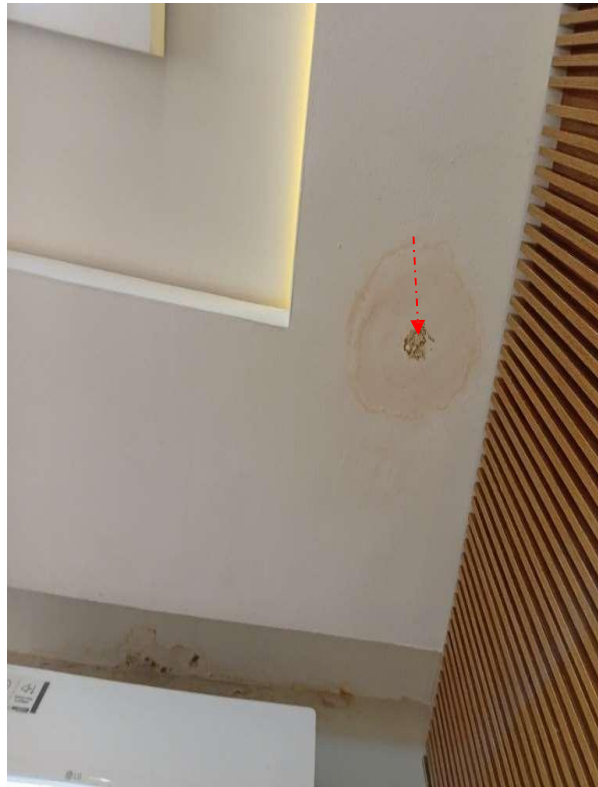
Pic showing the visible appearance of Pop discolouration due to water leakage from the Master bedroom terrace
