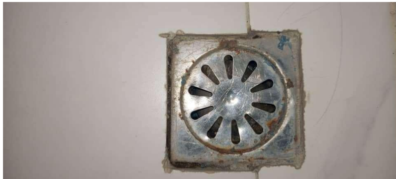
Pic Showing: Corroded floor drain with deteriorated sealant around the drain frame, indicating maintenance and resealing are required.
