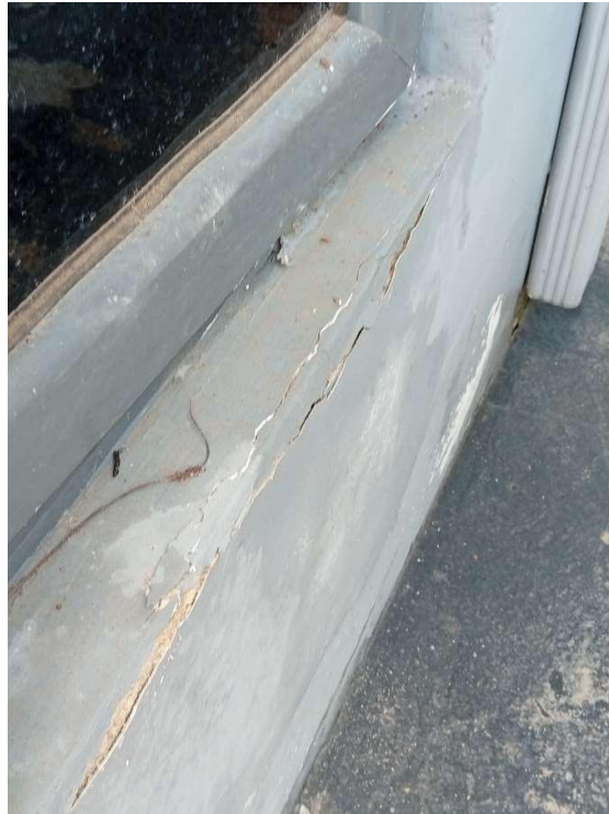
Pics showing flaky walls from base foundation attributed to severe rising damp or water intrusion.
