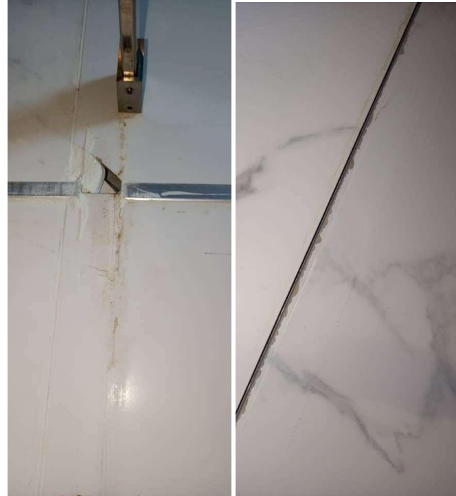
Pic showing: Displacement of Metal tile trim / divider.
