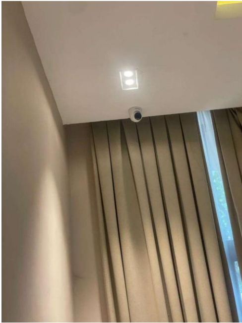
Picture showing a properly installed CCTV camera internally
