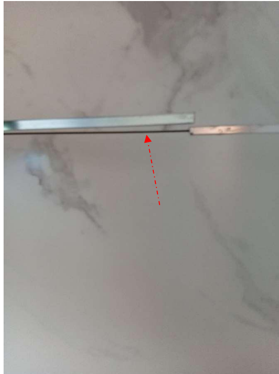
Pic showing: Displacement of metal tile trim / divider due to poor installation or thermal expansion.
