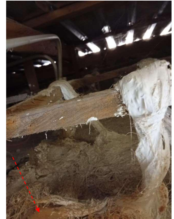
Pic showing: The wood members of the roofing systems being attacked by termites, causing the wood to deteriorate and lose its strength.
