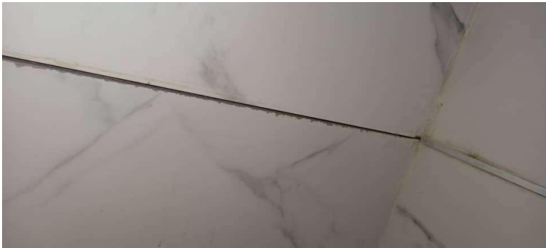
Pic showing: Displacement of Metal tile trim/divider.
