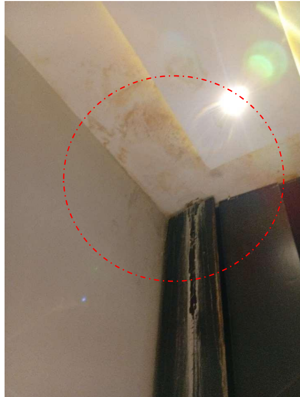
Pic showing: Pop discoloration due to water leakage from the master bedroom open terrace floor.
