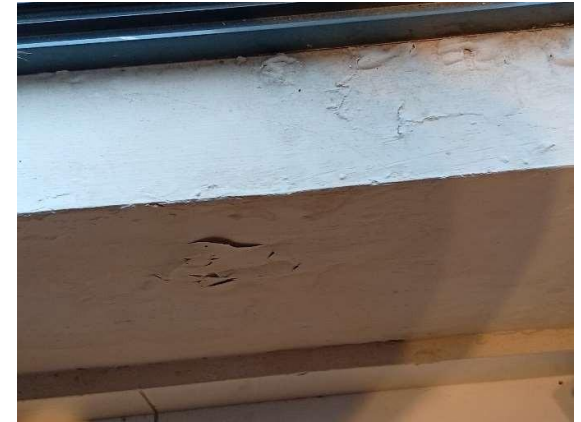
Pic showing water ingress into the wall from window level, making the area of the block wall damp.
