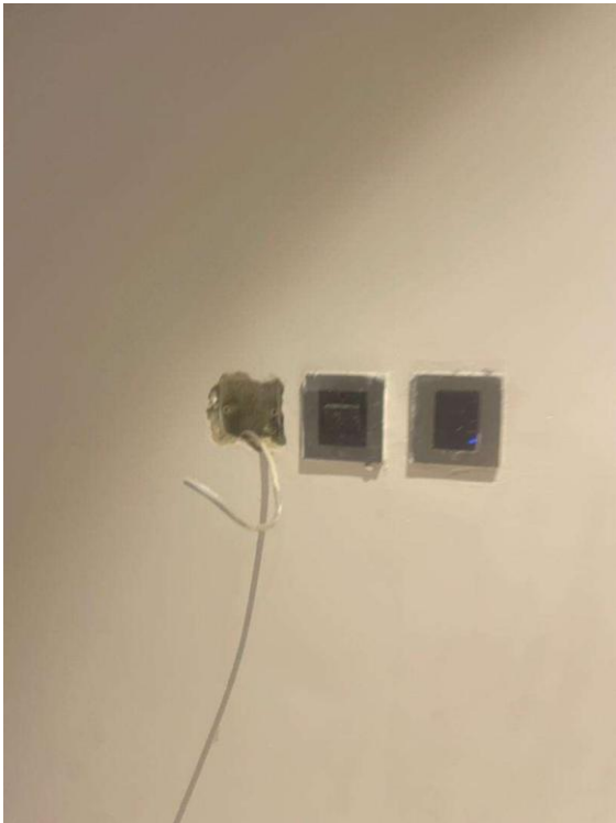
Picture showing exposed recess box
