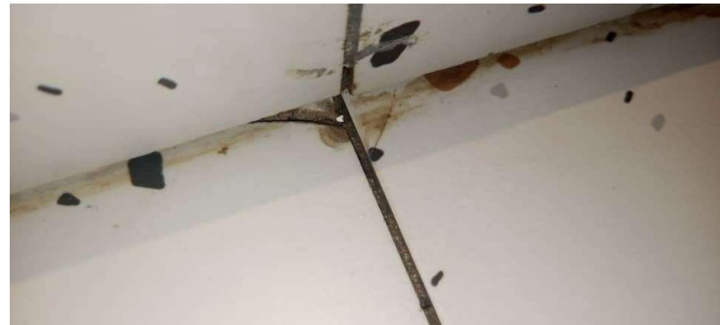
Pic showing: Toilet floor and wall tiles with Poor grouting
