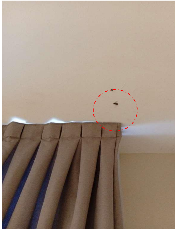
Pic showing: Punctured holes on the Pop ceiling board may indicate poor finishing or workmanship quality.
