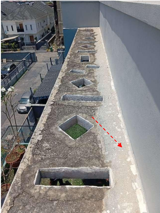
Pics showing a poorly cast afterthought roof slab, sand, and cement patch characterized by multiple porous holes, which have permitted water ingress into the underlying floor slab. This condition has consequently compromised the structural integrity of the slab.
