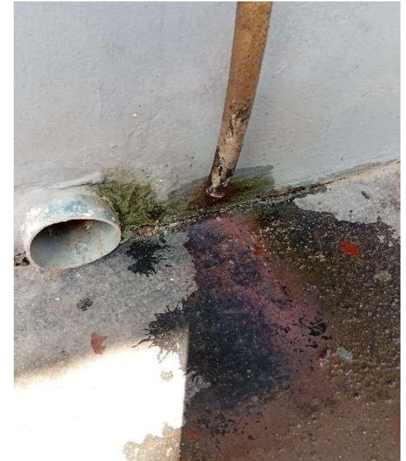
Pics showing water discharge from Ac outdoor unit making the wall edges turn greenish.
